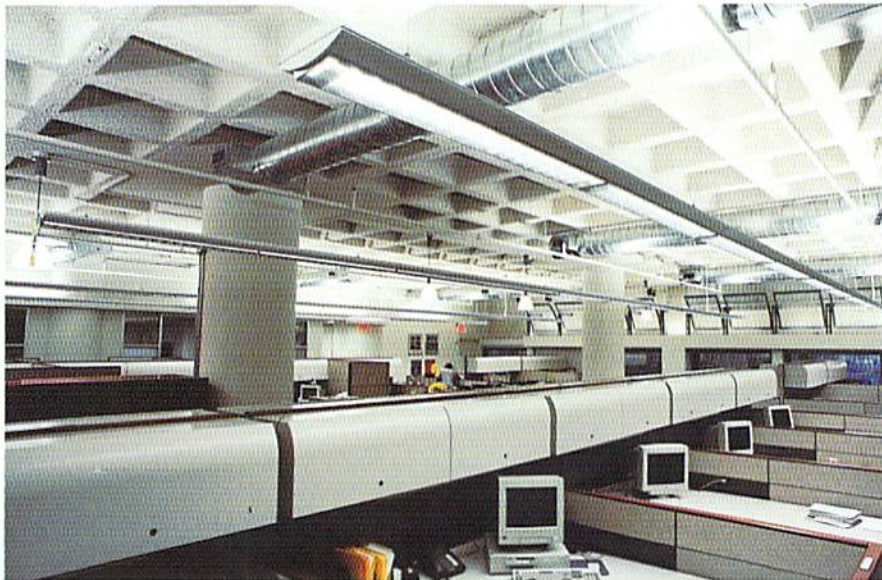
Thirteen/WNET, New York, New York Architect: HLW International Acoustical Consultant: Shen Milsom & Wilke
